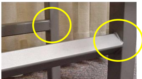
Fig. 11. The square tubing on the left will accumulate soil on the flat horizontal surface. By rotating 90°, or using round tubing, flat surfaces are minimized.
